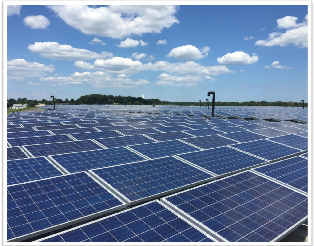
Brick Solar Field - Sally Ike Rd., Township of Brick, Ocean County
